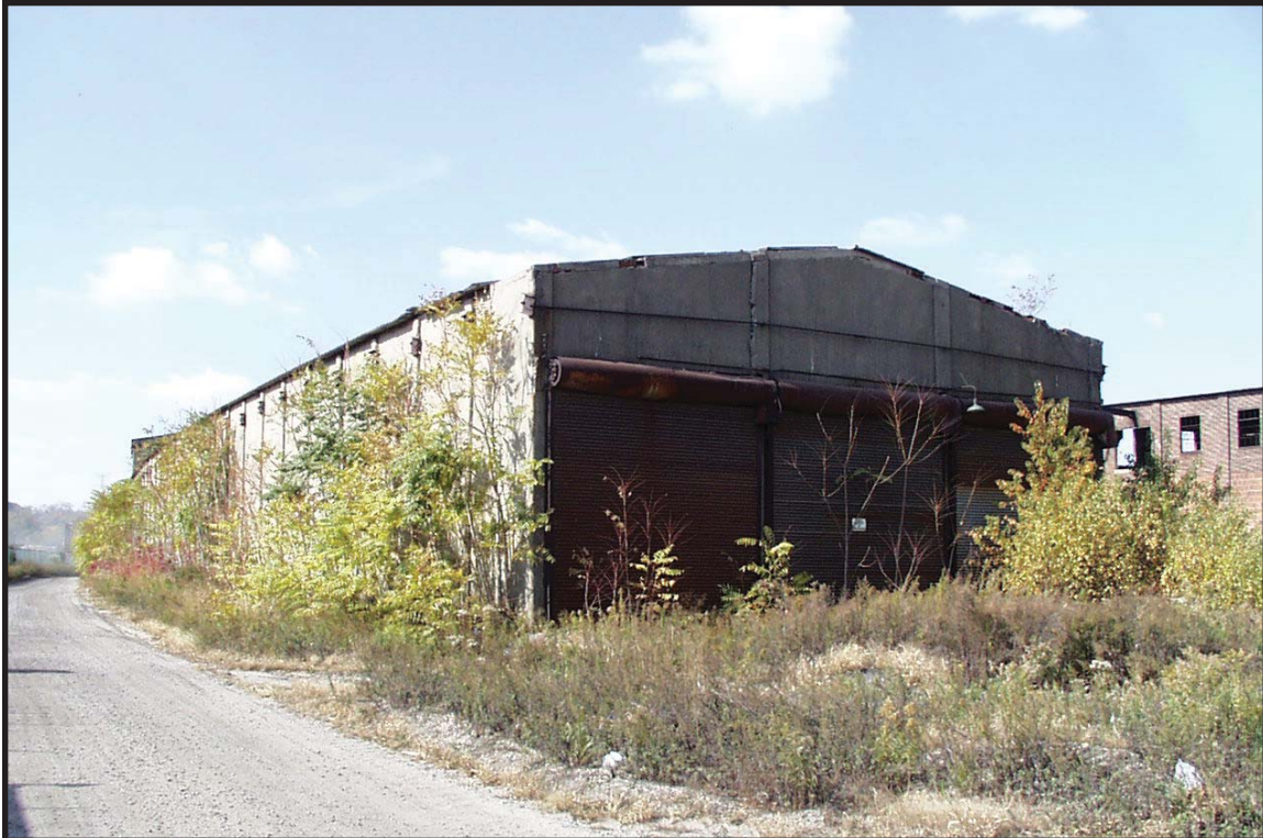
Photograph 6.5. View looking west-northwest showing the eastern end of the 1916 shed, with part of the 1911 shed visible at right (Photographer: Ian Burrow, October 2001) [HRI Neg. #01005/D3:13].
