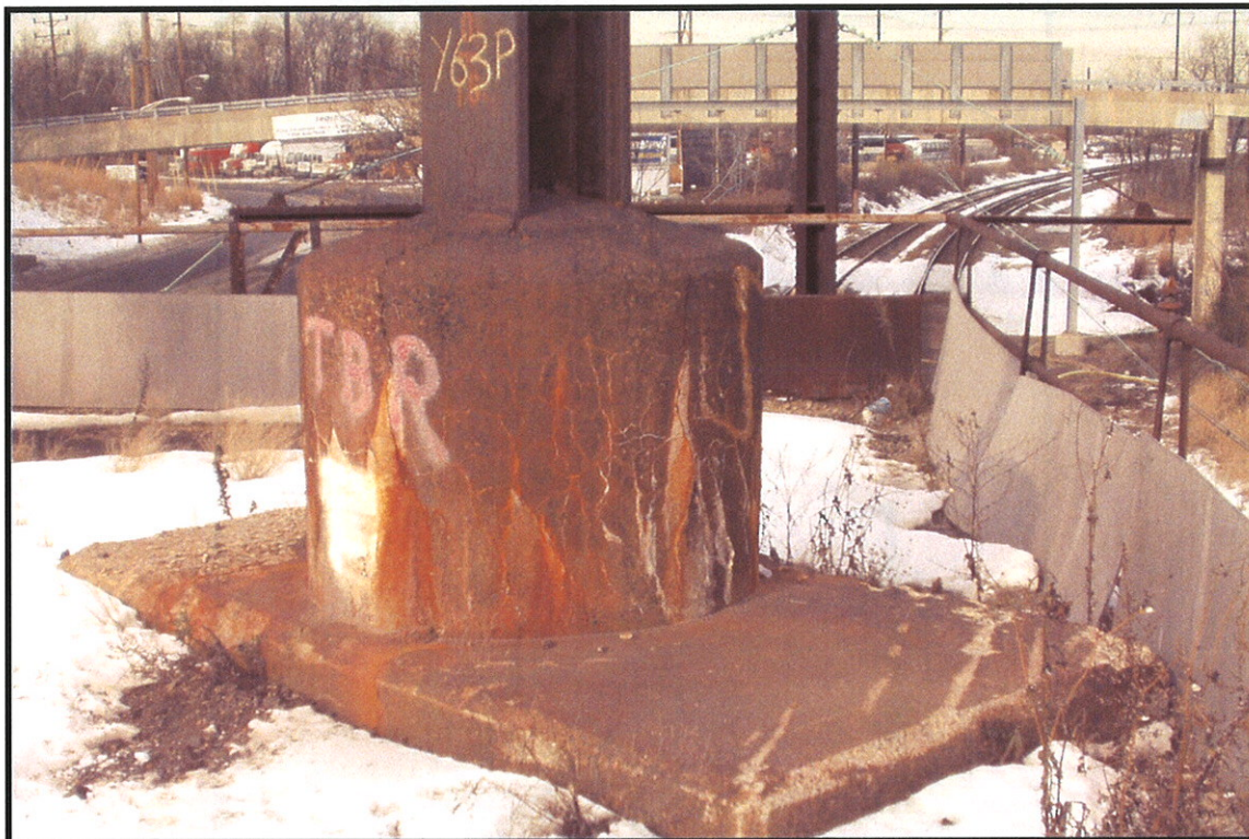
Plate 3. The base of Portal Bridge Catenary C10a from the southeast, showing concrete slab mat and concrete pedestal typical of Pennsylvania Railroad construction (Photographer: Ian Burrow, December 2002). [Hunter Research Inc. Negative 02081/D1:03].
