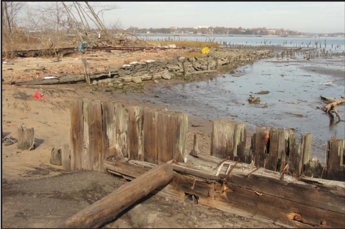
Photograph 7.12. View looking north-northeast showing the timber and stone revetment probably placed after 1950 to stabilize the shoreline after the 1950 explosion that destroyed the explosives pier. The stones include a number of Camden and Amboy Railroad-era stone sleepers which should be salvaged and used for interpretive purposes at the new ferry terminal (Photographer: Ian Burrow, October 2012) [HRI Neg. #11027/D5:DSC03614].
