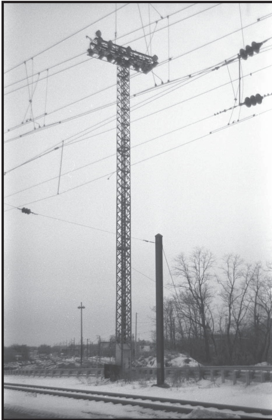
Photograph 5.38. Light pole at the South Amboy ferry terminal (Photographer: Ian Burrow, 2002) [HRI Neg. # 02081/1:08].
