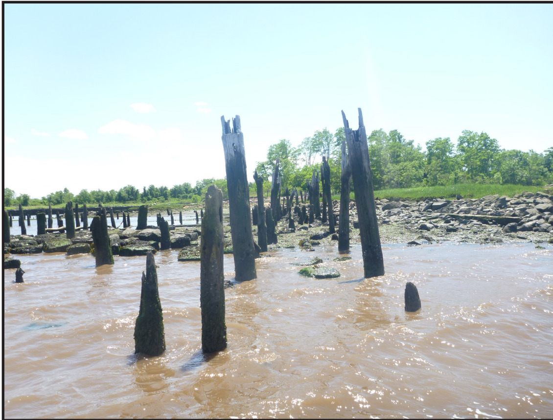
Photograph 3.6. View looking southwest along the line of the catwalk connecting the barge rack to the shore. Note that many of the walkway piles are taller than those supporting the adjoining deck to the left. Some of these piles may also be remnants of the New Brunswick Pier, built in 1891 and continuing in place until circa 1920 when the barge rack and catwalk were constructed (Photographer: Joshua Butchko, June 2019) [HRI Neg.# 19013/D1:075].
