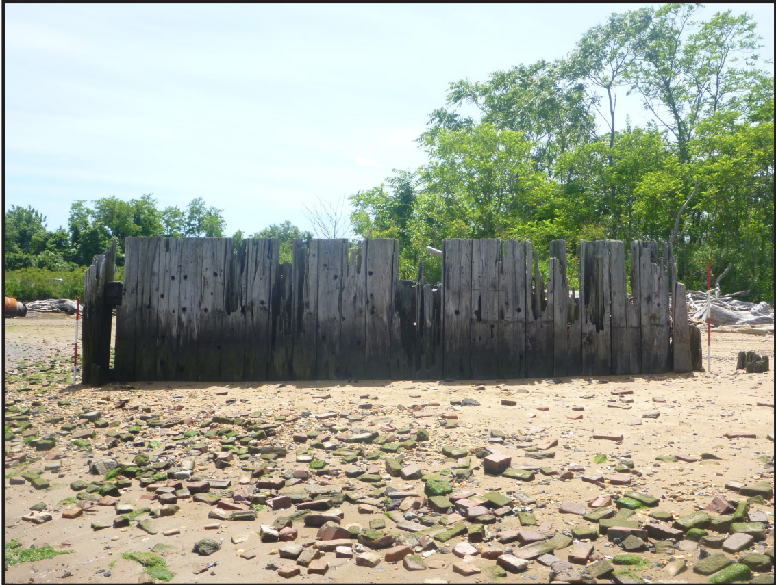
Photograph 3.33. Detailed view looking southeast along the interior of the short segment of bulkhead from which the explosives pier, built in the mid-1920s, projected out into Raritan Bay. This view shows the close-set, vertical timber pile, transverse timber and “dead man” construction of the bulkhead, which may originally date from the early 1870s and be contemporary with the Westmoreland and Lehigh piers. The Westmoreland Pier is across the water at the top of the view (Photographer: Joshua Butchko, June 2019) [HRI Neg.# 19013/D1:213].
