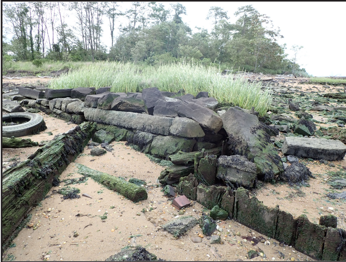
Photograph 3.26. View looking west showing a section of railroad embankment with a stone retaining wall along its southeastern face. The embankment appears to have transitioned at this point to a timber trestle supported on piles and sheeting. These remains may date from the Pennsylvania Railroad era in the early 1870s or possibly from a mid-19th-century expansion of the freight terminal during the Camden and Amboy Railroad era (Photographer: James Lee, September 2020) [HRI Neg.# 19013/D10:064].
