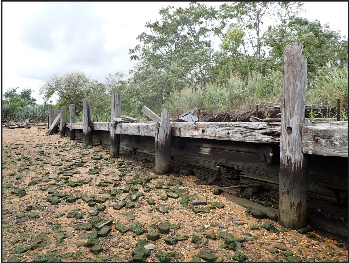
Photograph 3.35. View looking west showing the vertical timber pile and transverse beam construction of the long segment of bulkhead extending southwest from the base of the explosives pier. This section of bulkhead may originally date from the early 1870s and be contemporary with the Westmoreland and Lehigh piers. Note that some of the transverse timbers are flush with the front of the piles, probably indicating docking locations (Photographer: James Lee, September 2020) [HRI Neg.# 19013/D10:075].
