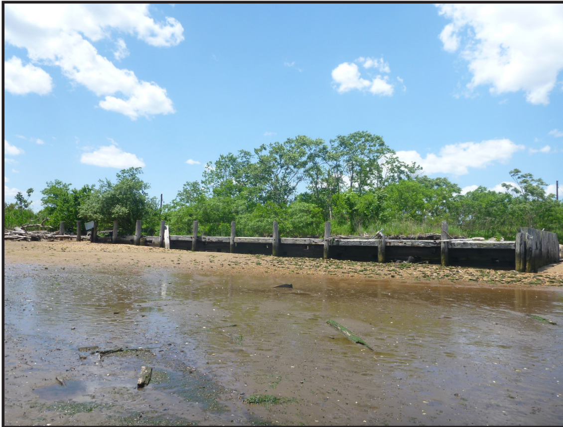
Photograph 3.34. View looking west showing the southeast face of the long segment of bulkhead extending southwest from the base of the explosives Pier. This section of bulkhead may originally date from the early 1870s and be contemporary with the Westmoreland and Lehigh piers. The short bulkhead segment is at right (Photographer: Joshua Butchko, June 2019) [HRI Neg.# 19013/D1:041].
