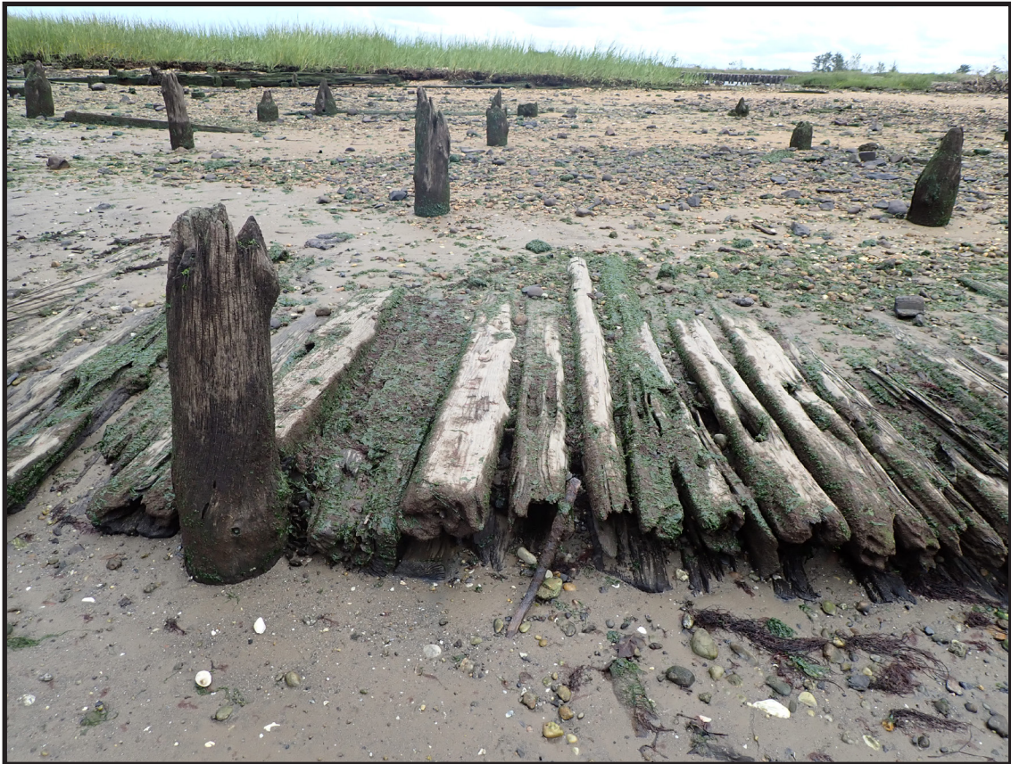
Photograph 3.9. View looking southeast showing the northwestern edge of the timber corduroy ramp. The ramp is composed of a single layer of horizontally laid, sawn and rough-hewn timbers, each roughly ten feet long, laid side by side on the bay floor (Photographer: James Lee, September 2020) [HRI Neg.# 19013/D10:023].
