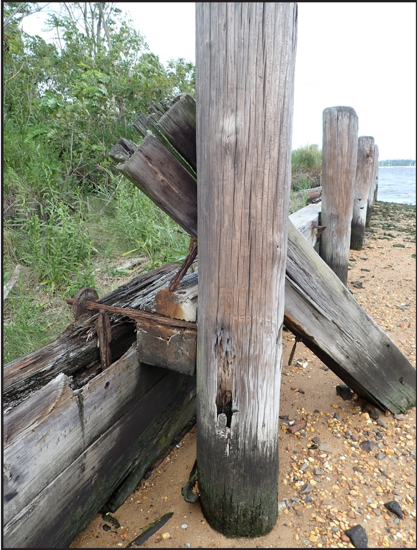
Photograph 3.36. Detailed view looking north showing the mode of construction of the long segment of bulkhead extending southwest from the base of the explosives pier. Note the piles are offset from the bulkhead wall and the bulkhead components are bolted and spiked together with iron hardware (Photographer: James Lee, September 2020) [HRI Neg.# 19013/D10:076].
