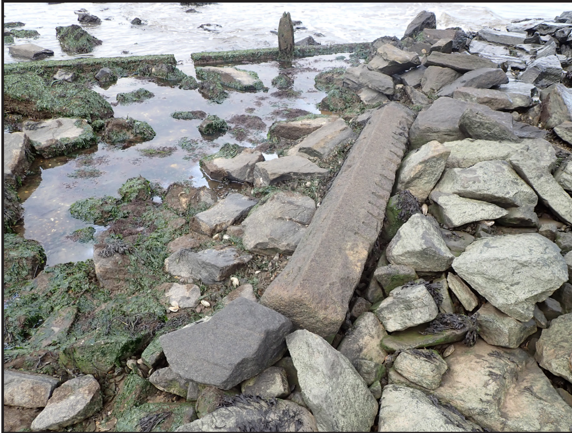
Photograph 3.27. View looking northeast showing the northeastern end of the main stone retaining wall/bulkhead with a large stone sill in the center of the view. The horizontal timber beam and vertical pile at upper left are part of an angled section of timber cribbing that runs east-west between the retaining wall and the nearby railroad embankment. These features may date from the Pennsylvania Railroad era in the early 1870s or possibly from a mid-19th-century expansion of the freight terminal during the Camden and Amboy Railroad era. They would have supported the rail approaches to the freight terminal (Photographer: James Lee, September 2020) [HRI Neg.# 19013/D10:072].
