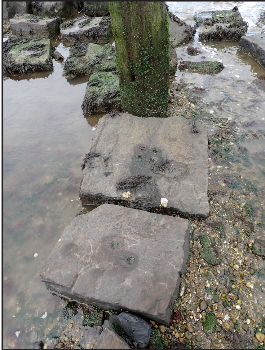
Photograph 3.21. View looking northeast showing typical two-hole and four-hole stone sleepers placed against one of the piles of Piling Structure B (Photographer: James Lee, September 2020) [HRI Neg.# 19013/D10:039].
