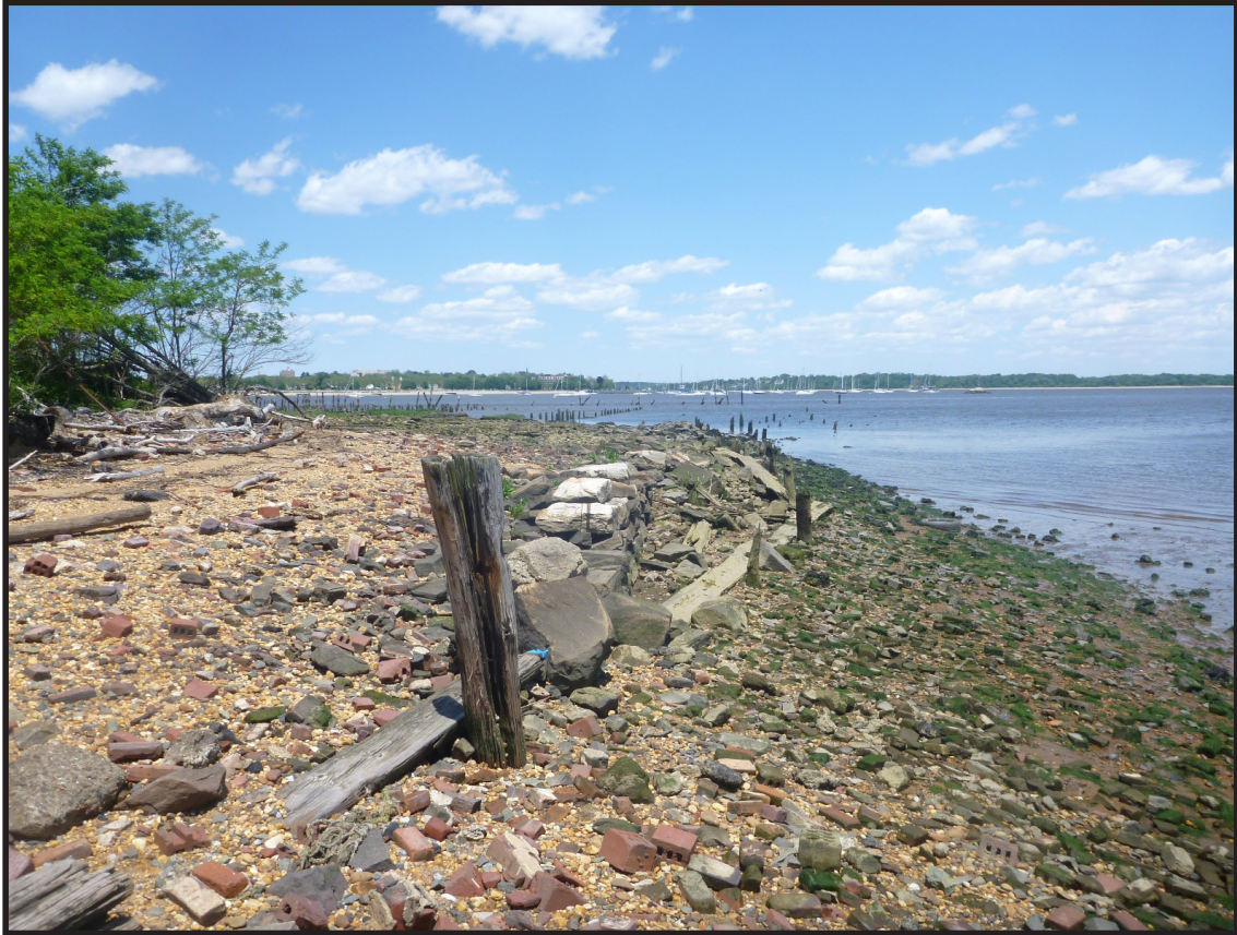
Photograph 3.29. View looking northeast along the retaining wall/bulkhead that defines the southeastern edge of the Camden and Amboy Railroad/Pennsylvania Railroad freight terminal. The transverse timbers and vertical piles of the bulkhead lining the southeastern face of the stone retaining wall may be a later modification; the retaining wall is thought to date from the Pennsylvania Railroad era in the early 1870s or possibly from a mid-19th-century expansion of the freight terminal during the Camden and Amboy Railroad era. The large square stone blocks are sleepers re-used from the Camden and Amboy Railroad rail beds (Photographer: Joshua Butchko, June 2019) [HRI Neg.# 19013/D1:050].
