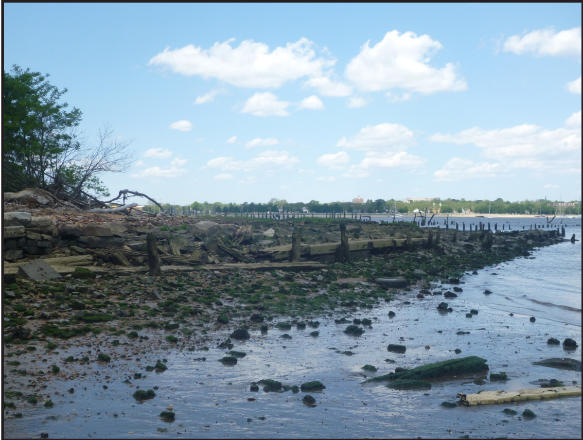
Photograph 3.28. View looking north towards the retaining wall/bulkhead that defines the southeastern edge of the Pennsylvania Railroad freight terminal. The transverse timbers and vertical piles of the bulkhead lining the southeastern face of the stone retaining wall may be a later modification; the retaining wall is thought to date from the Pennsylvania Railroad era in the early 1870s or possibly from a mid-19th-century expansion of the freight terminal during the Camden and Amboy Railroad era (Photographer: Joshua Butchko, June 2019) [HRI Neg.# 19013/D1:049].
