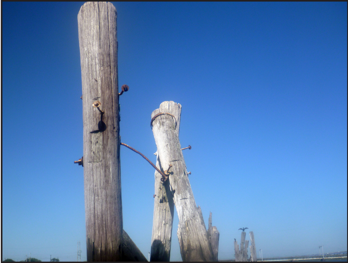
Photograph 3.3. View looking west-northwest showing examples of the barge rack piles with iron hardware (spikes, bolts, nuts, washers and bands) (Photographer: Joshua Butchko, August 2019) [HRI Neg.# 19013/D7:060].
