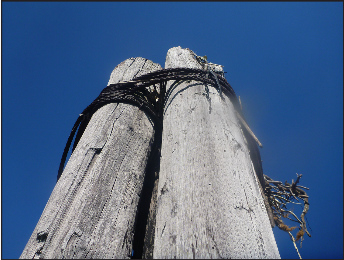
Photograph 3.4. Close-up view of a typical cluster pile, comprised of multiple logs bound together with wire rope and iron staples, at the northwestern end of the barge rack (Photographer: Joshua Butchko, August 2019) [HRI Neg.# 19013/D7:040].
