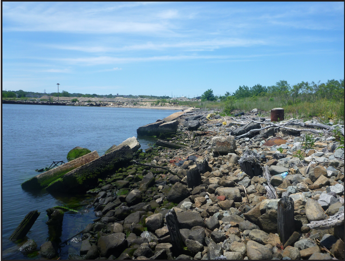
Photograph 3.45. Lehigh Pier: view looking southwest along the southern edge of the pier. Erosion has revealed fill material (Photographer: Joshua Butchko, June 2020) [HRI Neg.# 19013/D8:046].
