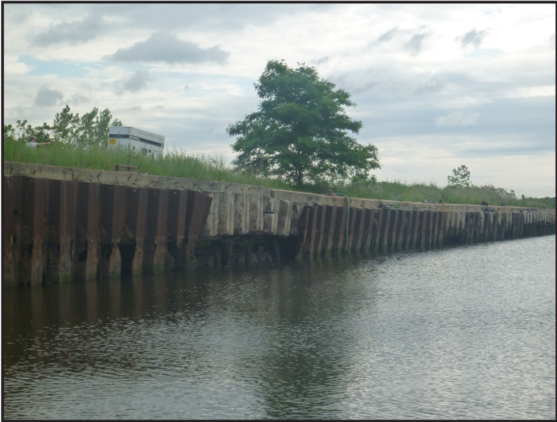
Photograph 3.44. Lehigh Pier: view looking northeast at the southwestern end of the pier. The steel Z-sheet piles have fallen away at spots revealing concrete caps and the older timber piles and sheeting of the pier’s original fender system (Photographer: Joshua Butchko, June 2020) [HRI Neg.# 19013/D8:024].
