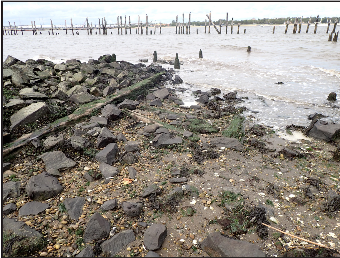
Photograph 3.17. View looking northwest showing the eastern end of the promontory. The long horizontal beam marks the southeastern side of a bulkhead apparently encasing the tip of the promontory, upon which is piled rock fill. These remains are interpreted as dating from the Camden and Amboy Railroad era, possibly from the early 1830s. The barge rack is in the middle distance (Photographer: James Lee, September 2020) [HRI Neg.# 19013/D10:035].
