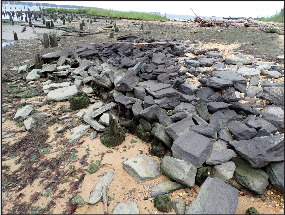
Photograph 3.7. View looking northeast showing the bulkhead and rock fill at the northwestern end of the project site. Note the vertical timber piles in front of the timber plank sheeting retaining the rock fill and defining the exterior face of the bulkhead. The piles beyond relate to Piling Structure A, considered to be part of a mid-19th-century expansion of the Camden and Amboy Railroad, while the original early 1830s Camden and Amboy Railroad wharf straddled the grassy promontory in the distance (Photographer: James Lee, September 2020) [HRI Neg.# 19013/D10:017].
