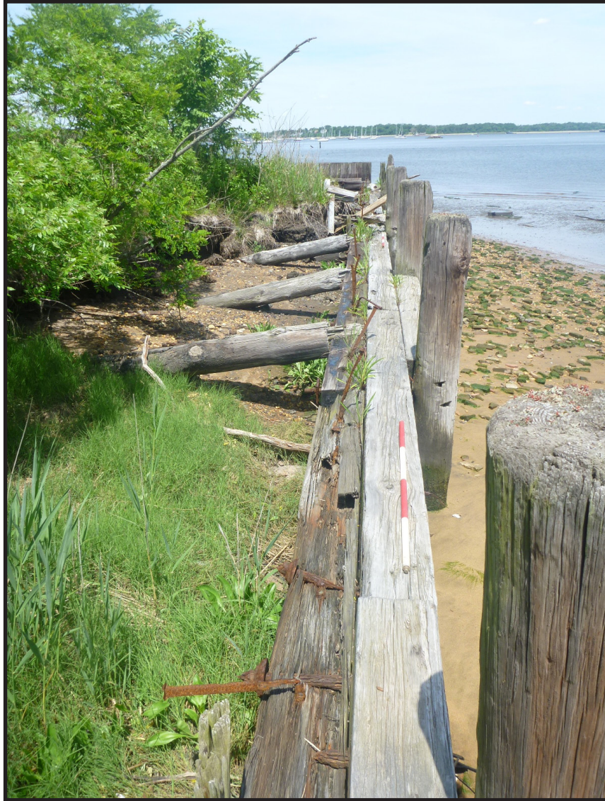
Photograph 3.37. View looking northeast along the line of the long segment of bulkhead extending southwest from the base of the explosives pier. Note the mode of construction making use of vertical piles, transverse timbers and “dead man” bracing fastened with iron bolts and spikes. Scale in feet (Photographer: Joshua Butchko, June 2019) [HRI Neg.# 19013/D1:192].
