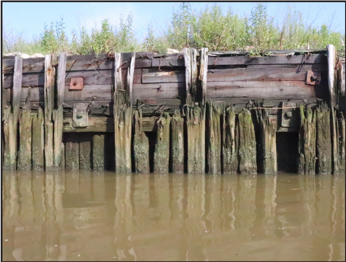
Photograph 3.40. Westmoreland Pier: view looking northwest at the southeast side of the pier showing timber sheet piles attached to horizontal timber runners to form the fender system (Photographer; Alexis Alemy, August 2019) [HRI Neg.# 19013/D3:316].
