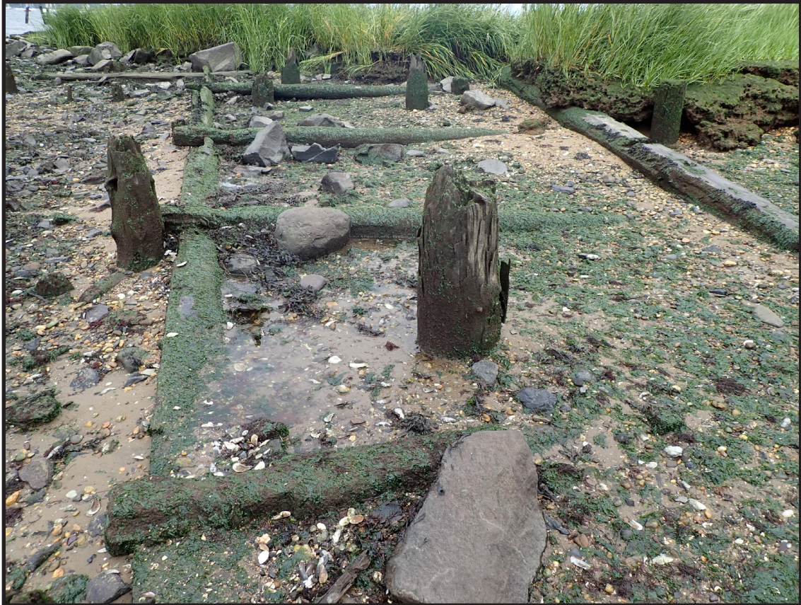
Photograph 3.12. View looking northeast along a section of timber bulkhead remains retaining the northwest side of the promontory. The large vertical timber piles, which pierce the bulkhead, are part of Piling Structure A. This bulkhead is interpreted as dating from the Camden and Amboy Railroad era, possibly from the early 1830s (Photographer: James Lee, September 2020) [HRI Neg.# 19013/D10:027].
