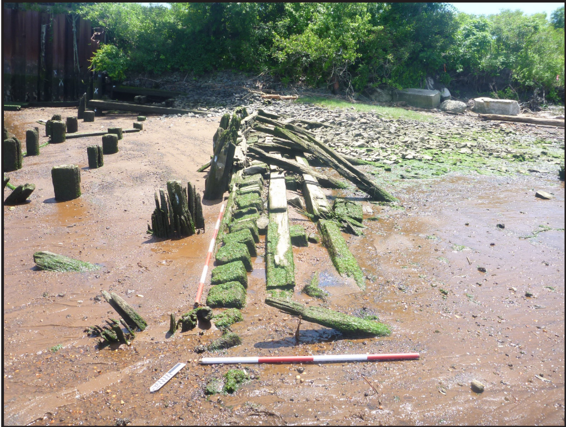
Photograph 3.42. View looking southeast at remnant timber bulkhead at the southwestern end of the slip between the Westmoreland and Lehigh piers (Photographer: Joshua Butchko, June 2019) [HRI Neg.# 19013/D1:145].
